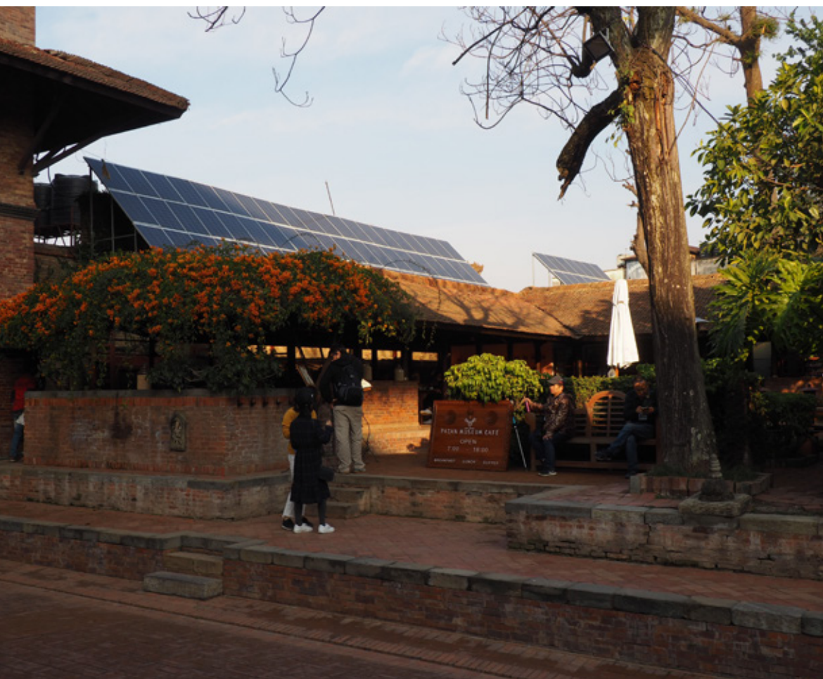
THE NEWLY INSTALLED SOLAR SYSTEM AT PATAN MUSEUM
